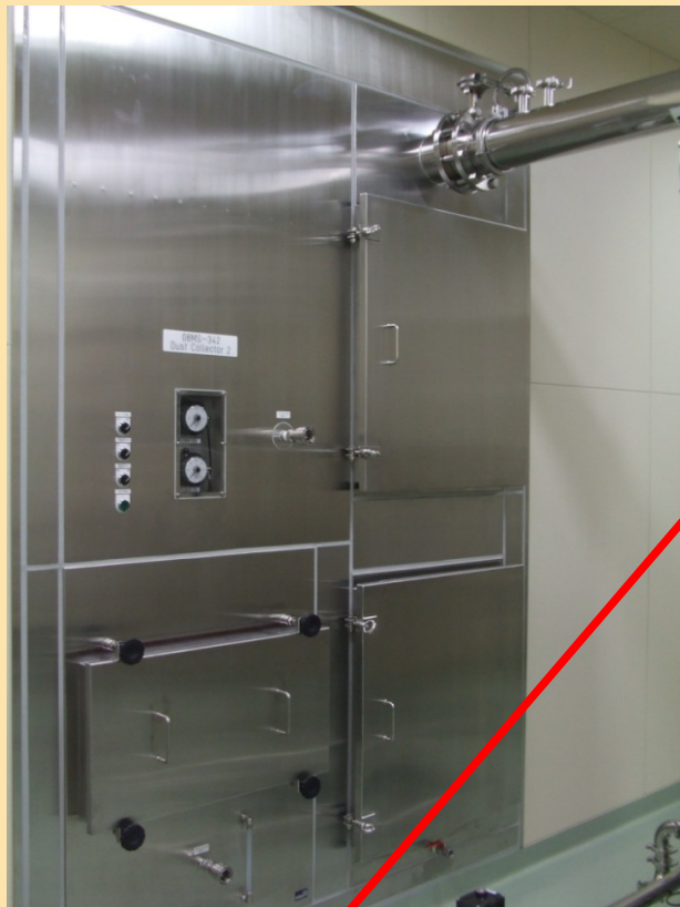
HEPA filter after dust collector
